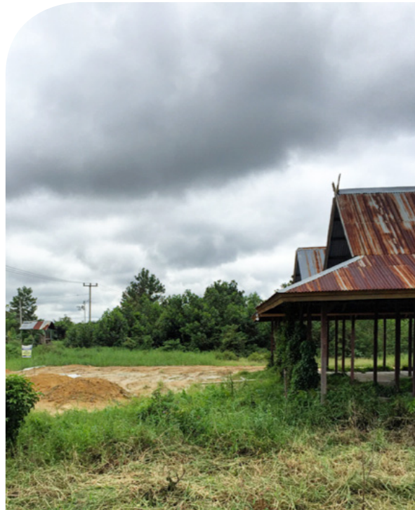
Currently the road is used as the market place resulting in traffic jams every Tuesday. However, once complete the market place will provide a stable trading platform that is a highly visible reward for FFVP when people come every week.
